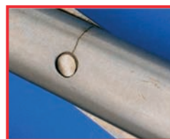
Fracture at hinge
